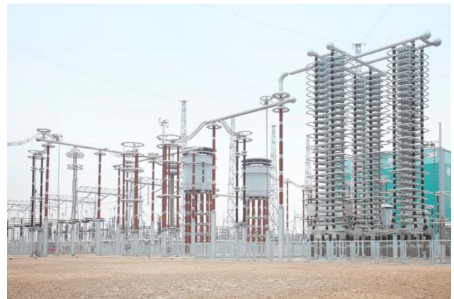
Fig. 3. Outdoor DC yard at Fengxiang station, XS800 project of SGCC
