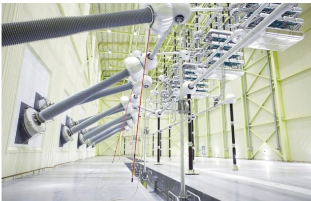
Fig. 7. HV valve hall at Fengxian station, XS800 project of SGCC
